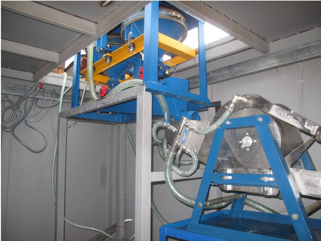
Wet magnetic separator MMS-2PM as part of the upgrading module DM-2
